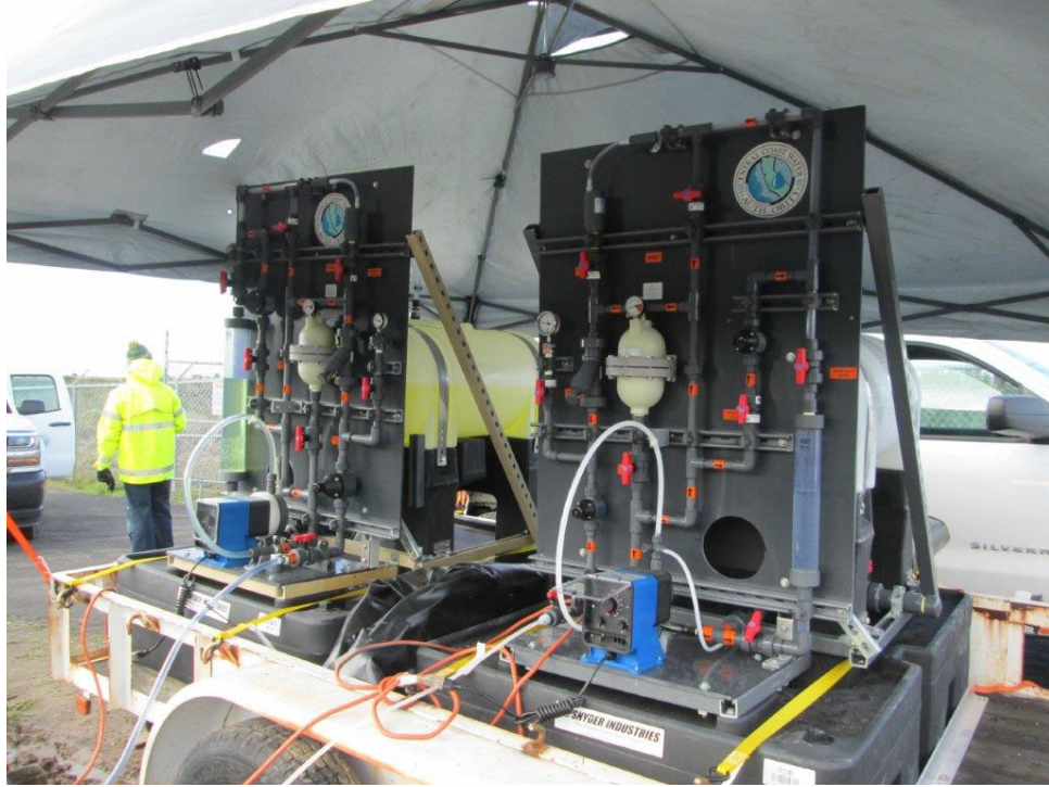
Tank 5 Inlet Vault Portable Chloramination Trailer, February 2022
