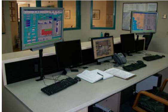
Treatment Plant Control Room
