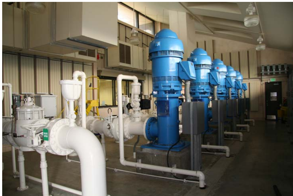
Santa Ynez Pumping Plant
