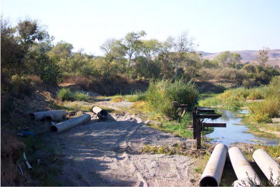
Exposed Pipeline Removal at the Santa Ynez River near Santa Rosa Road
