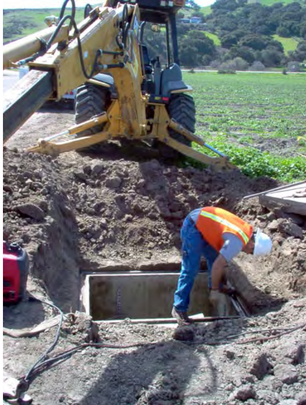
Distribution Technician, Jimmy Thompson, working at Fiber Optic Cable Splice Box on Drum Canyon Road
