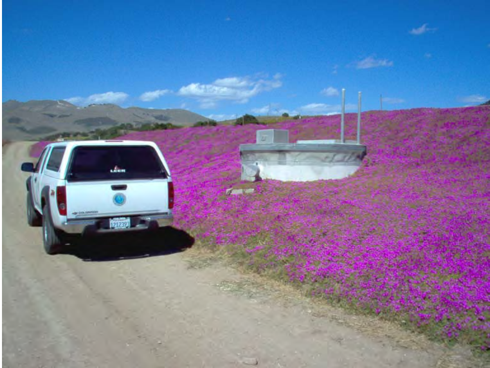
CCWA Valve Vault near Talley Farms in Arroyo Grande
