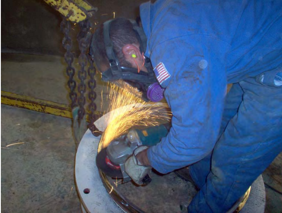
Distribution Supervisor, Tom Petersen, fitting the Dresser Coupling in the Outlet Meter Vault at the Santa Ynez Pump Station
