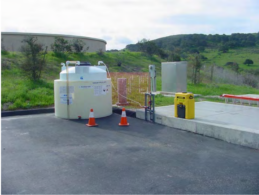
Tank 7 Temporary Chlorination Tank
