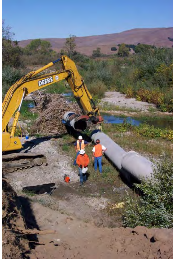
Contractor removing abandoned pipeline from the Santa Ynez River near Santa Rosa Road. This section was exposed during a flood event in the spring of 2001
