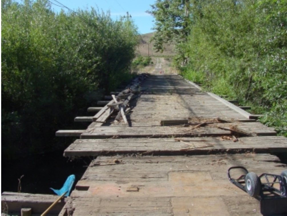
Above: Arroyo Grande bridge at the Arroyo Grande mitigation site during repairs completed in FY 2002/03.
