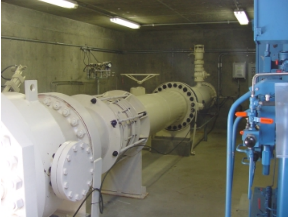
Above: Major blow-off valve at the Guadalupe turnout.
