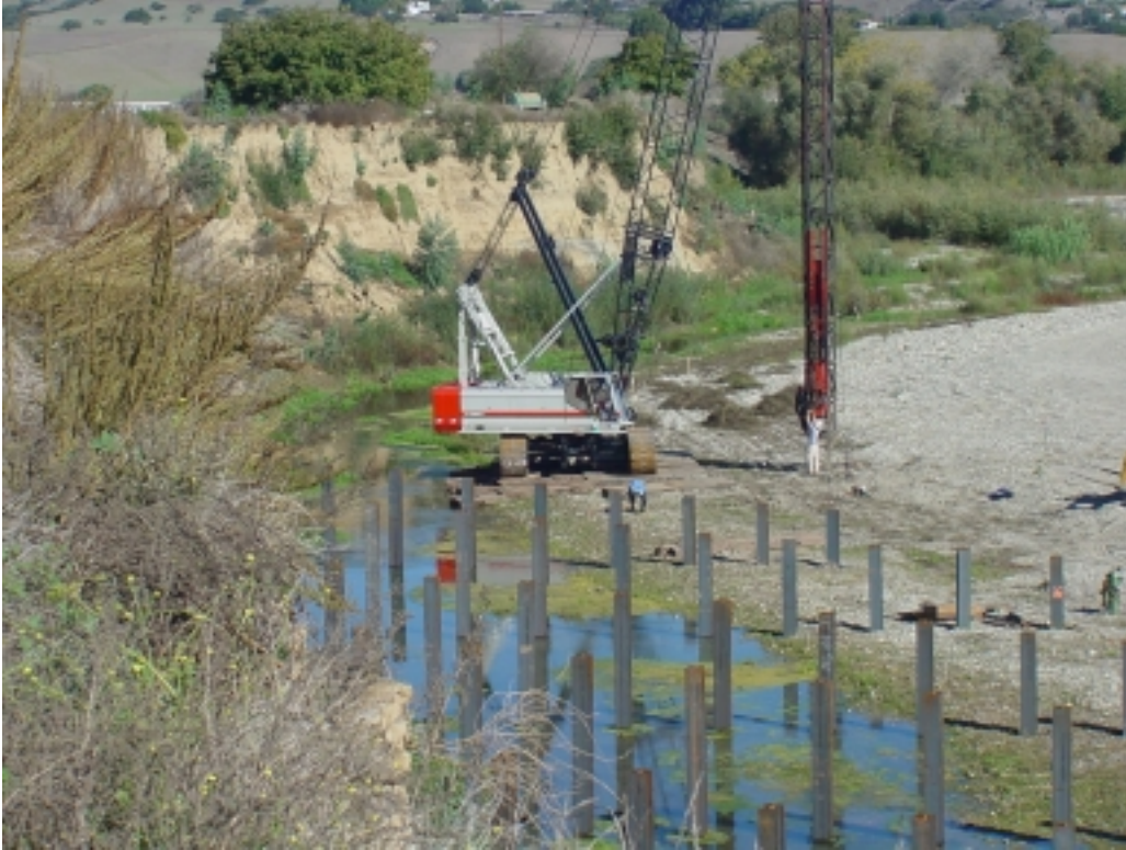
Above: Repairs to the CCWA pipeline which was exposed on the south side of the Santa Ynez River due to excessive rainfall and spill releases from Lake Cachuma in March 2001.
