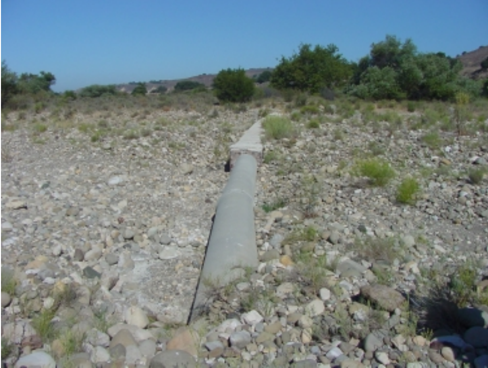
Above: Exposed CCWA pipeline at the Santa Ynez River, repaired during FY 2002/03.
