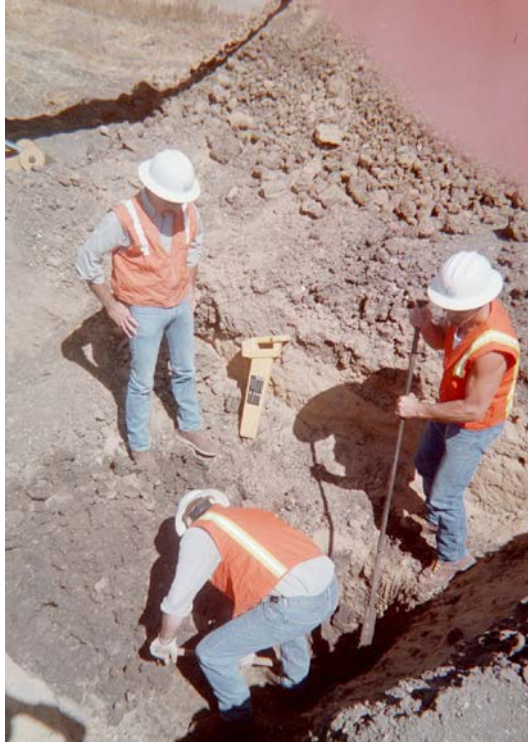
Above: CCWA Distribution staff inspecting welded pipe at Thompson Road in Nipomo.
