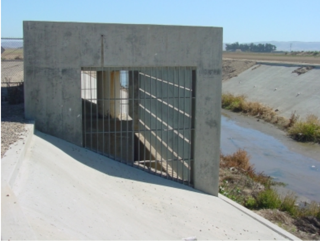
Above: Guadalupe turnout major blowoff structure used to drain the pipeline into the Santa Maria River.
