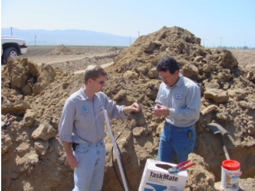
Above: Eric Kieding (left) and Woody Woodard (right) repair a broken section of the CCWA fiber optic cable downstream of the Southern California Water Company turnout.
