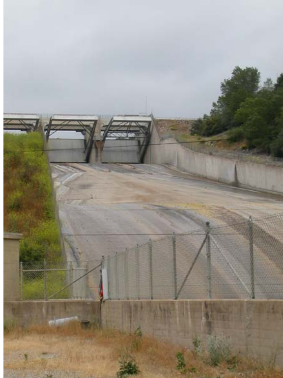
Above: Bradbury Dam spill-way into the Santa Ynez River from Lake Cachuma.
